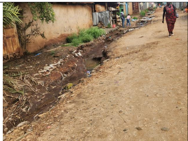
Unimproved earth road with poor storm water drainage infrastructure
